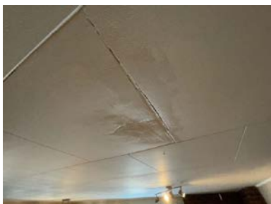
Skade i himling stue.
