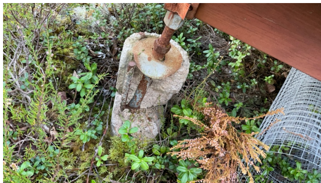
Dårlig betongfundament/pilar under ene platting.
