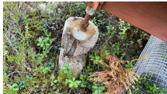
Dårlig betongfundament/pilar under ene platting.
