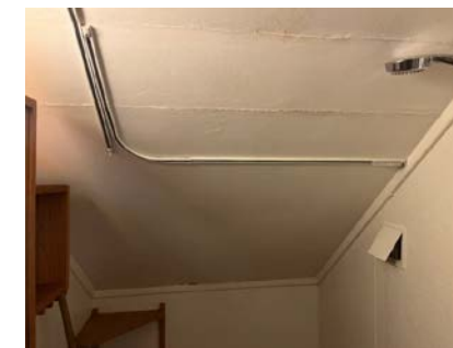
Sprekker i himling.
