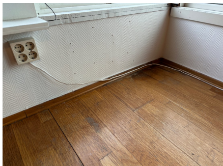
Eldre fuktmerker i parkett
