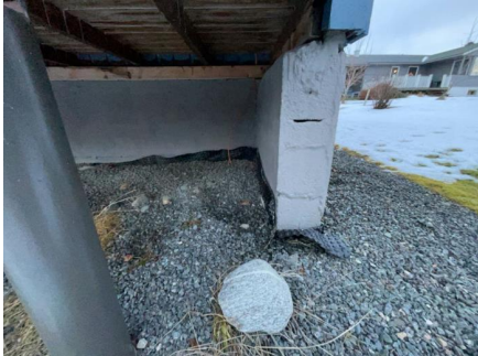
Mangler klemplatt under veranda
