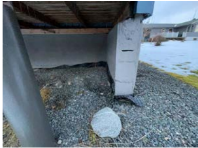
Mangler klemlist under veranda
