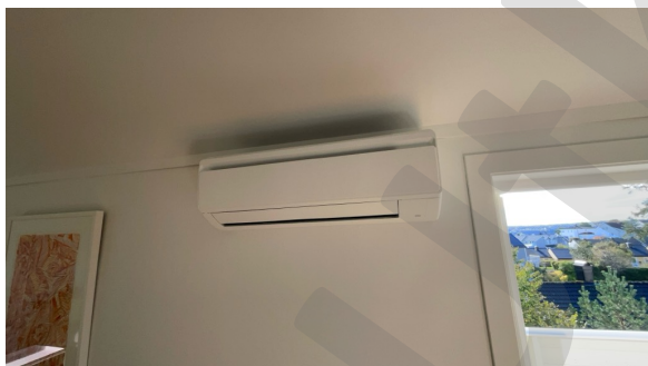
Varmepumpe, innvendig aggregat.
