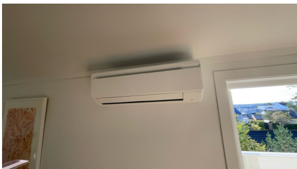
Varmepumpe, innvendig aggregat.
