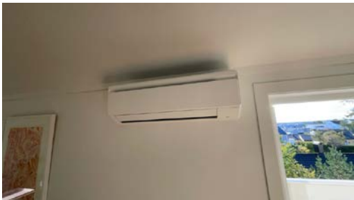
Varmepumpe, innvendig aggregat.
