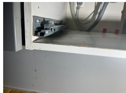
Fuktsvelling i bunnplate
