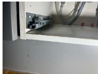
Fuktsvelling i bunnplate
