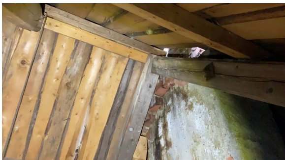
Manglende tetting rundt pipen.
