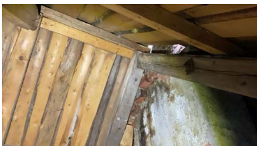
Manglende tetting rundt pipen.
