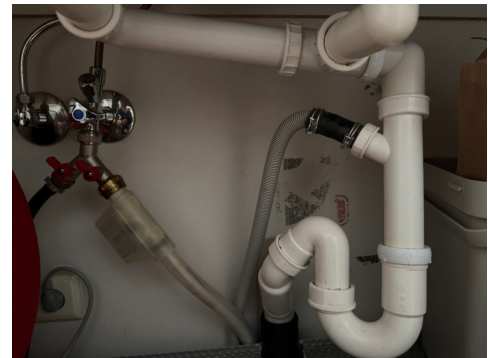
Røropplegg under vask.
