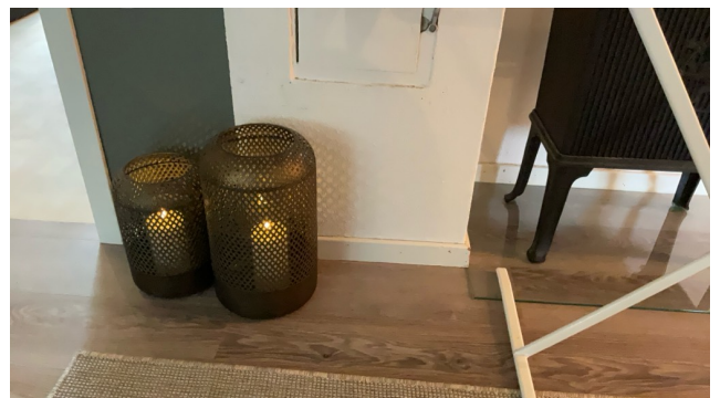
Ildfast plate under feieluke mangler.
