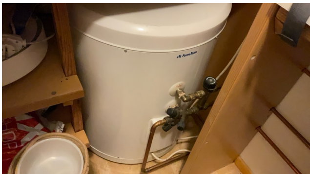
Bereder montert i bod.
