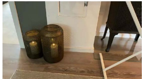
Ildfast plate under feieluke mangler.
