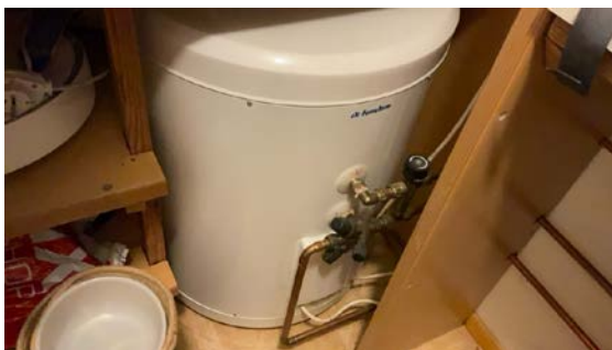
Bereder montert i bod.
