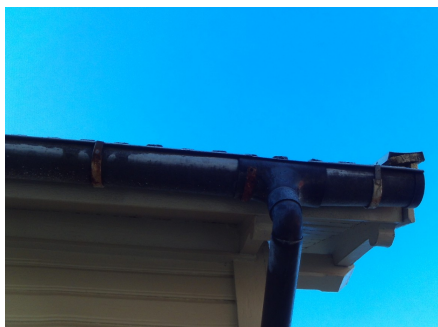
Eldre slitte takrenner
