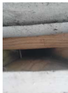
Manglende musesperre under kledning.
