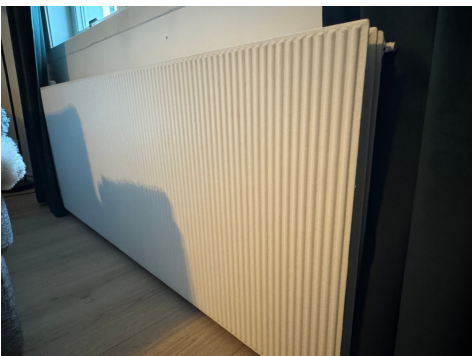
Eldre radiatorovn i stue.
