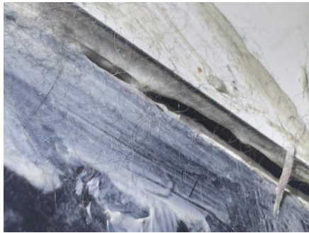
Manglende aluminiumslist under baderomsplatene.
