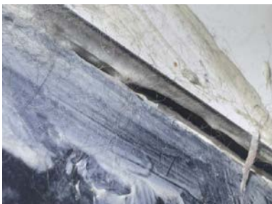
Manglende aluminiumslist under baderomsplaten.
