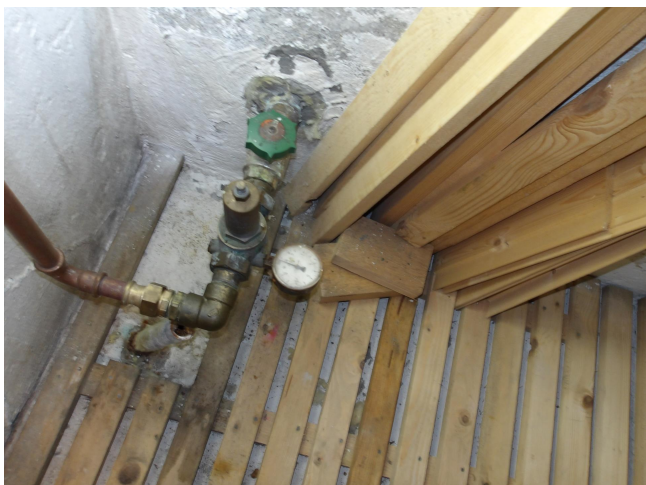
Stoppekran montert i bod.
