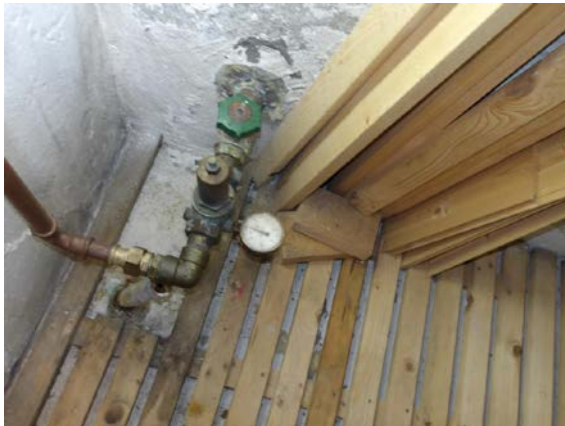
Stoppekran montert i bod.
