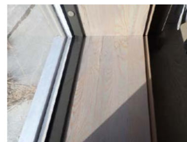
Sprekker i utforing.
