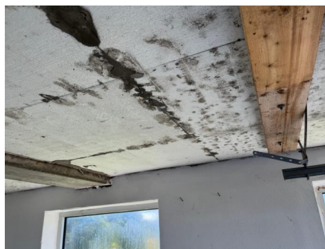
Synlig isopor i himling.
