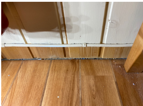
Stedvis manglende gulvlister.
