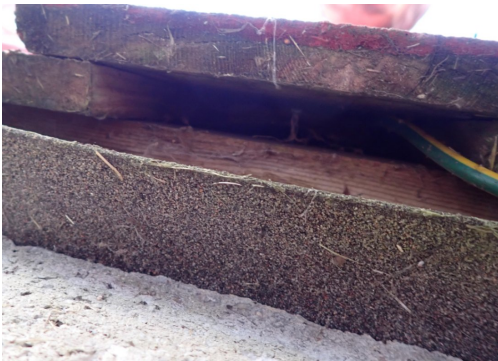
Viser manglende lusing/musesperre.
