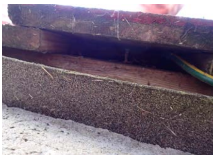
Viser manglende lusing/musesperre.
