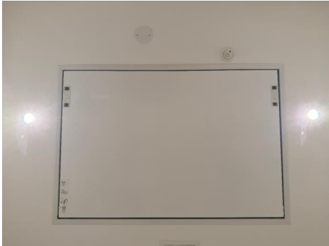
Luftbehandlingsaggregat i himling i entre/gang.
