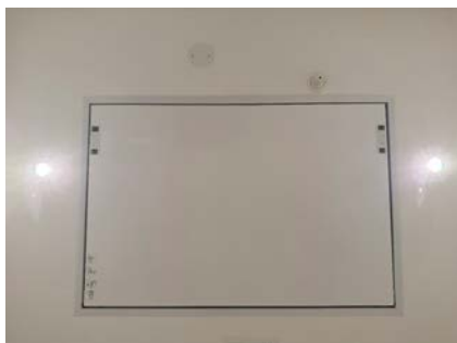
Luftbehandlingsaggregat i himling i entre/gang.
