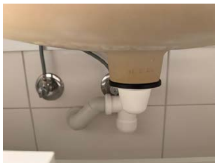
Røropplegg under servant.
